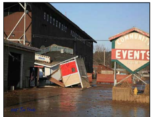
~Photo courtesy of Harry Green Damage at the Lewis County fairgrounds grandstand from the winter 2007 storm.
